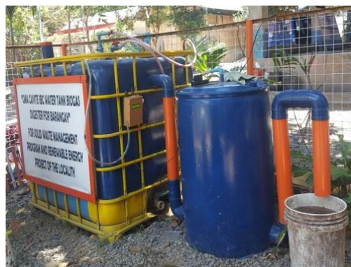
Figure 5. Device installed on the Biogas Digester
