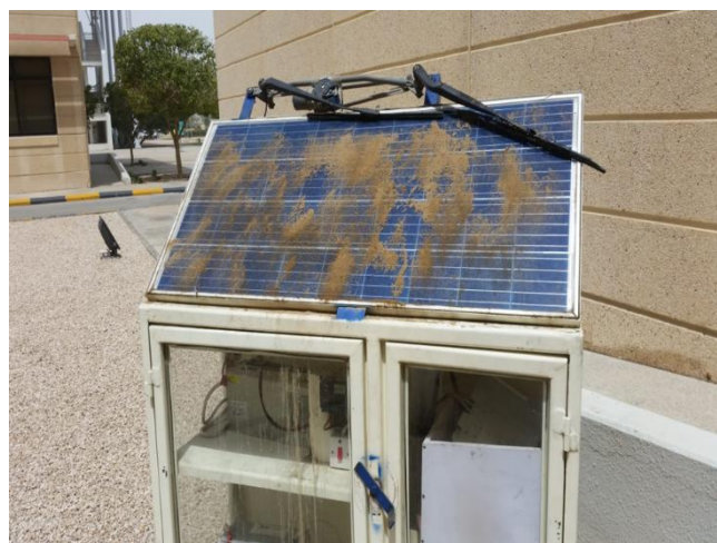
Fig. 4. Dust covering most area of the solar panel.
