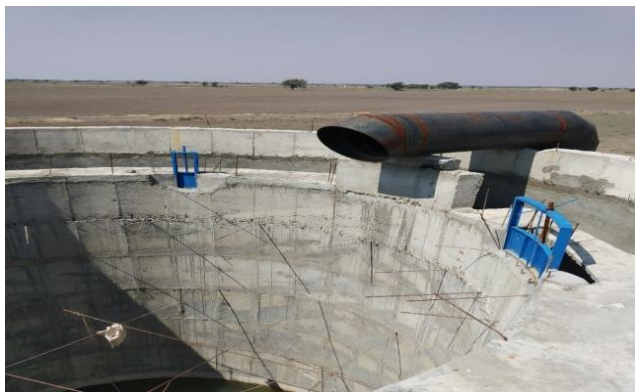
Figure 7: Main delivery cistern
